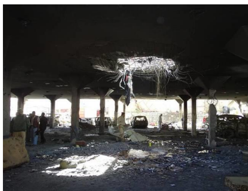
Figure 49.D.3 Post blast interior
